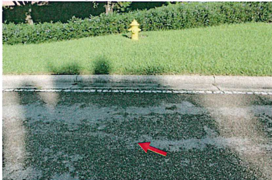
Missing Roadway Reflector
