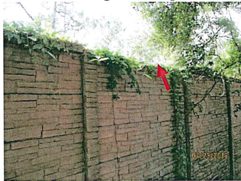
Missing Wall Cap
