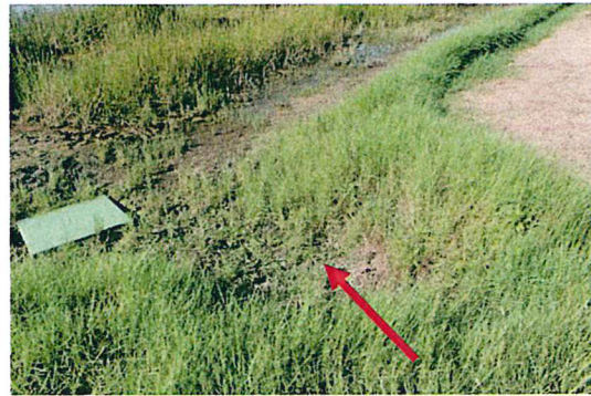
Washout on Lake 4
