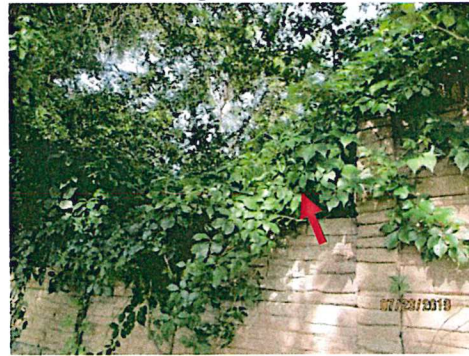
Missing Wall Panel
